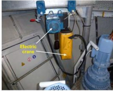
fig: electric hoist
